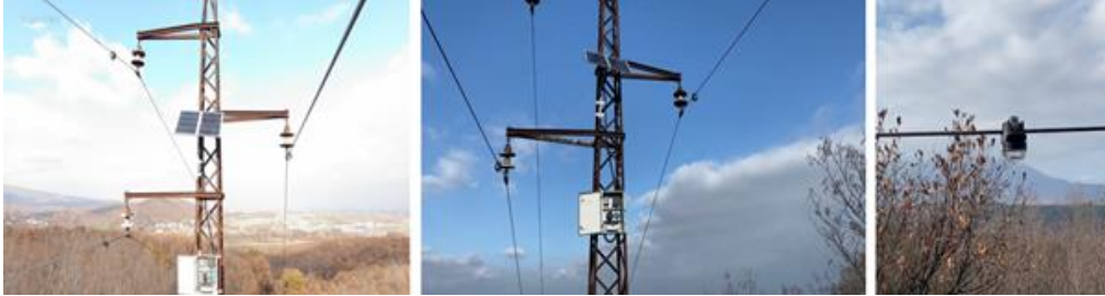
Fig. 1. Investigated 35 kV Prizreni 1–Zhuri overhead feeder corridor and installed fault passage indicator locations [32], [33]
