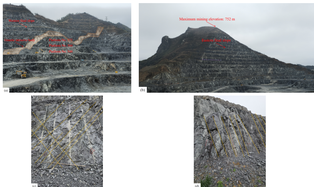
Fig. 2. Geotechnical conditions of the eastern and western slopes of the mine (a: West slope; b: East slope; c: Development of joints and fractures in the west slope; d: Development of joints and fractures in the east slope)
