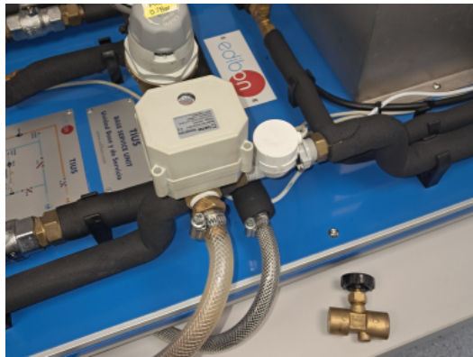
Fig. 3. Replacement of the manual heated-water valve with a proportional ball solenoid valve
