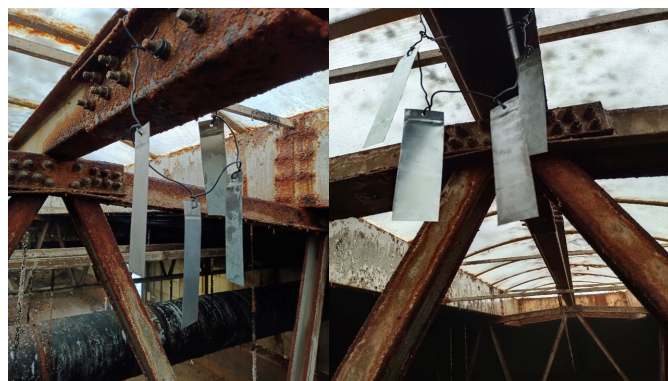
Figure 3. Steel and galvanized samples hung in the composting halls on the first day of exposure (2 steel and 2 galvanized).
