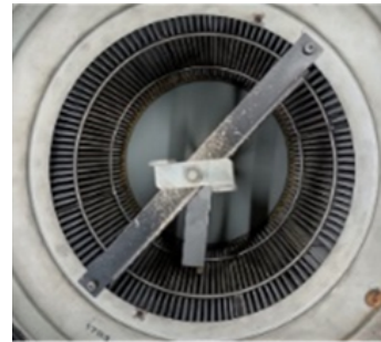
Fig. 6. Filter Dust Collector
