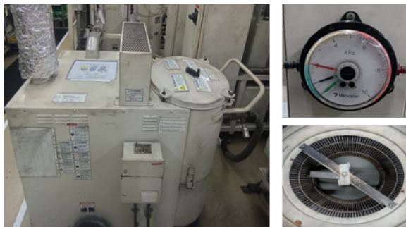
Fig. 14. Manual Dust Collector Condition without Warning
